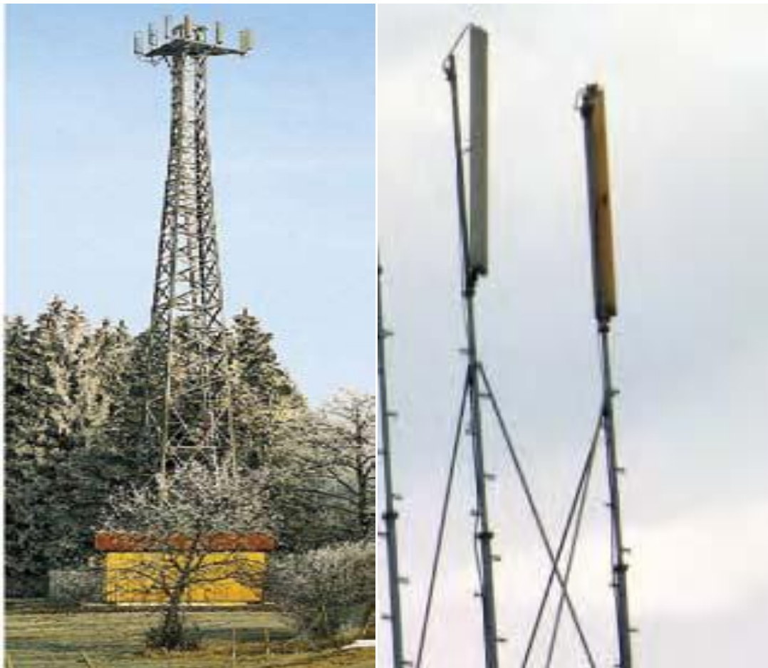
(a) A Transmission Tower
