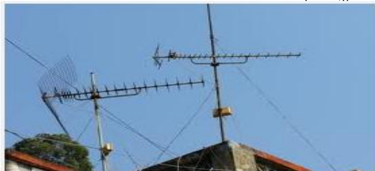
Figure 12: Yagi-Uda antenna placed on the roof.
